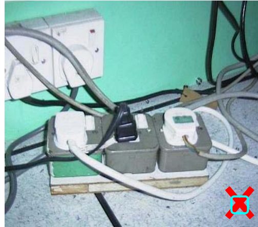
Haphazard electrical connections could lead to overloading and electrocution.
