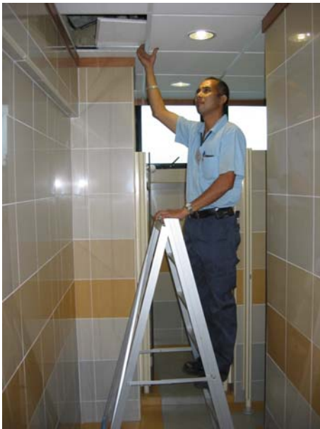
Use ladders safely
