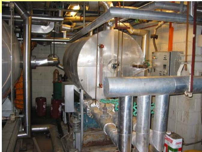
Boilers must be inspected regularly
