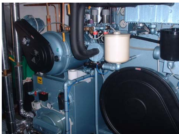
Dry cleaning machines must be maintained to prevent leakage of perchloroethylene
